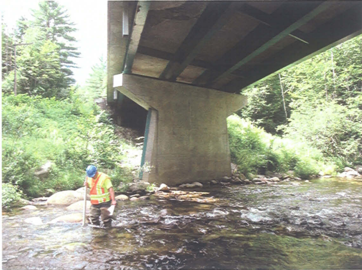
Scour Critical Feature at Low Water
