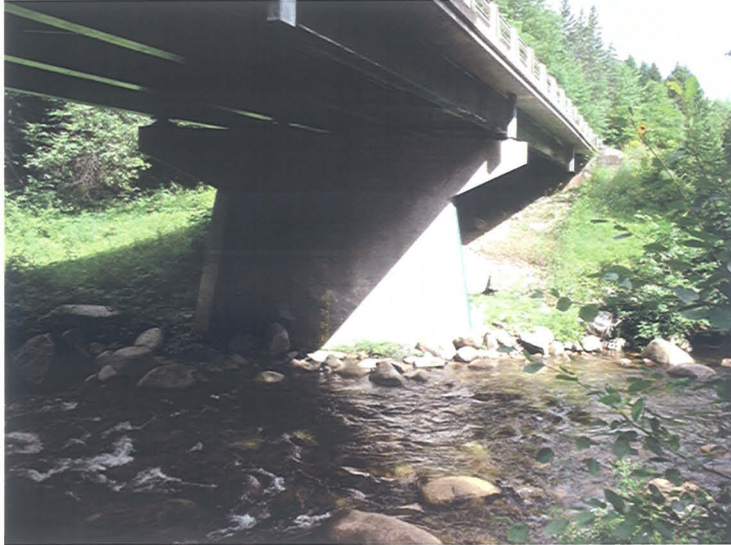
Scour Critical Feature at Low Water
